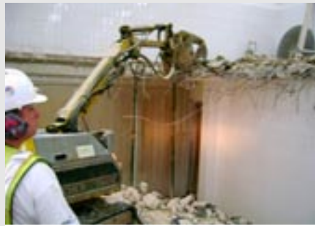
Hydraulic jaws on demolition robot crush out floor without noise or vibration.
