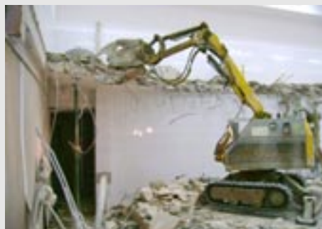
Brokk robot crushes out reinforced concrete floor in factory without disturbance to offices above
