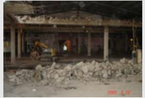
Brokk robot crushes large opening in roofslab to increase headroom of room
