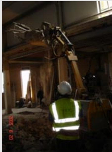
Robotic crusher breaks concrete structure to form opening without vibration and disruption to building occupiers
