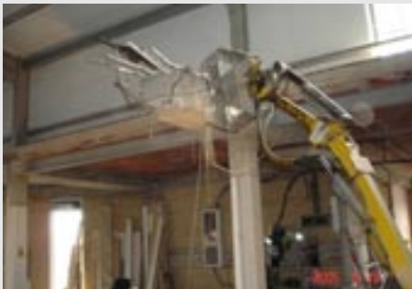
Demolition robot crushes reinforced concrete beam into rubble to form opening in floor slab
