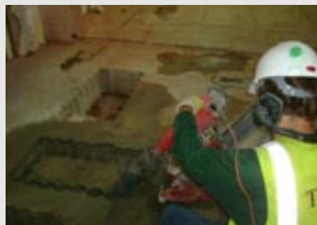
Vibration and dust free drilling of opening for cable entry to electric substation
